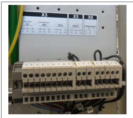
Figure 26. Alarm dry contacts
